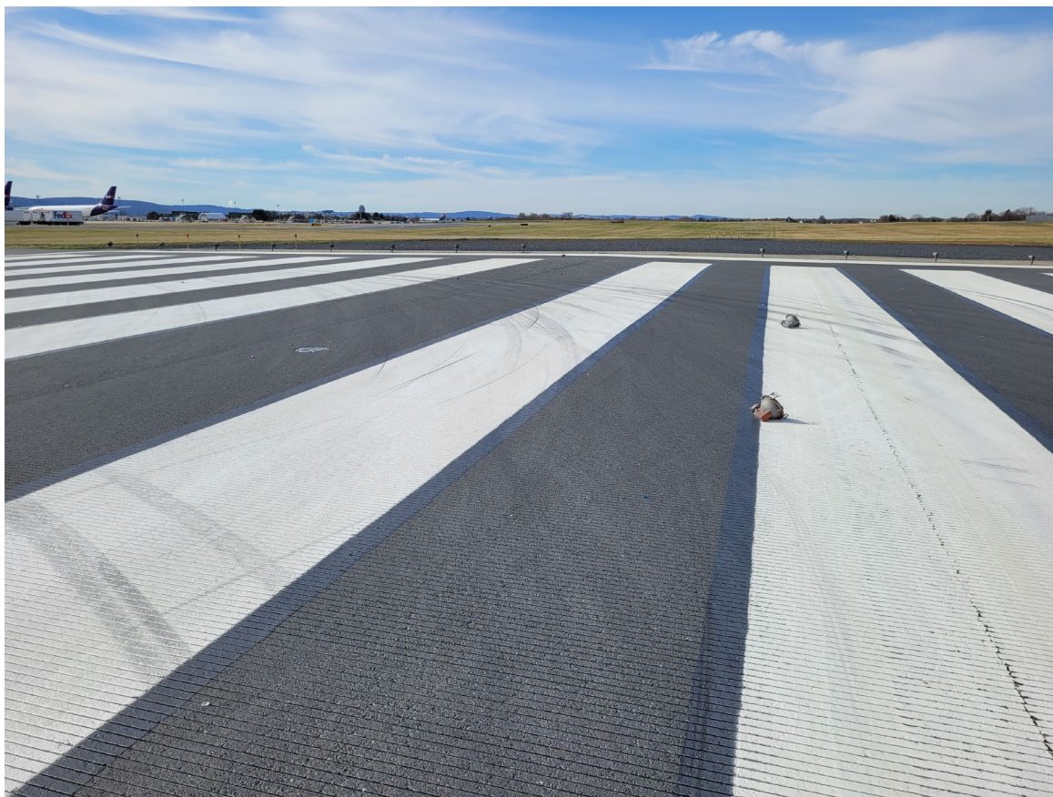
Photograph 4 - Runway Threshold Light Damage (Courtesy of FAA)
