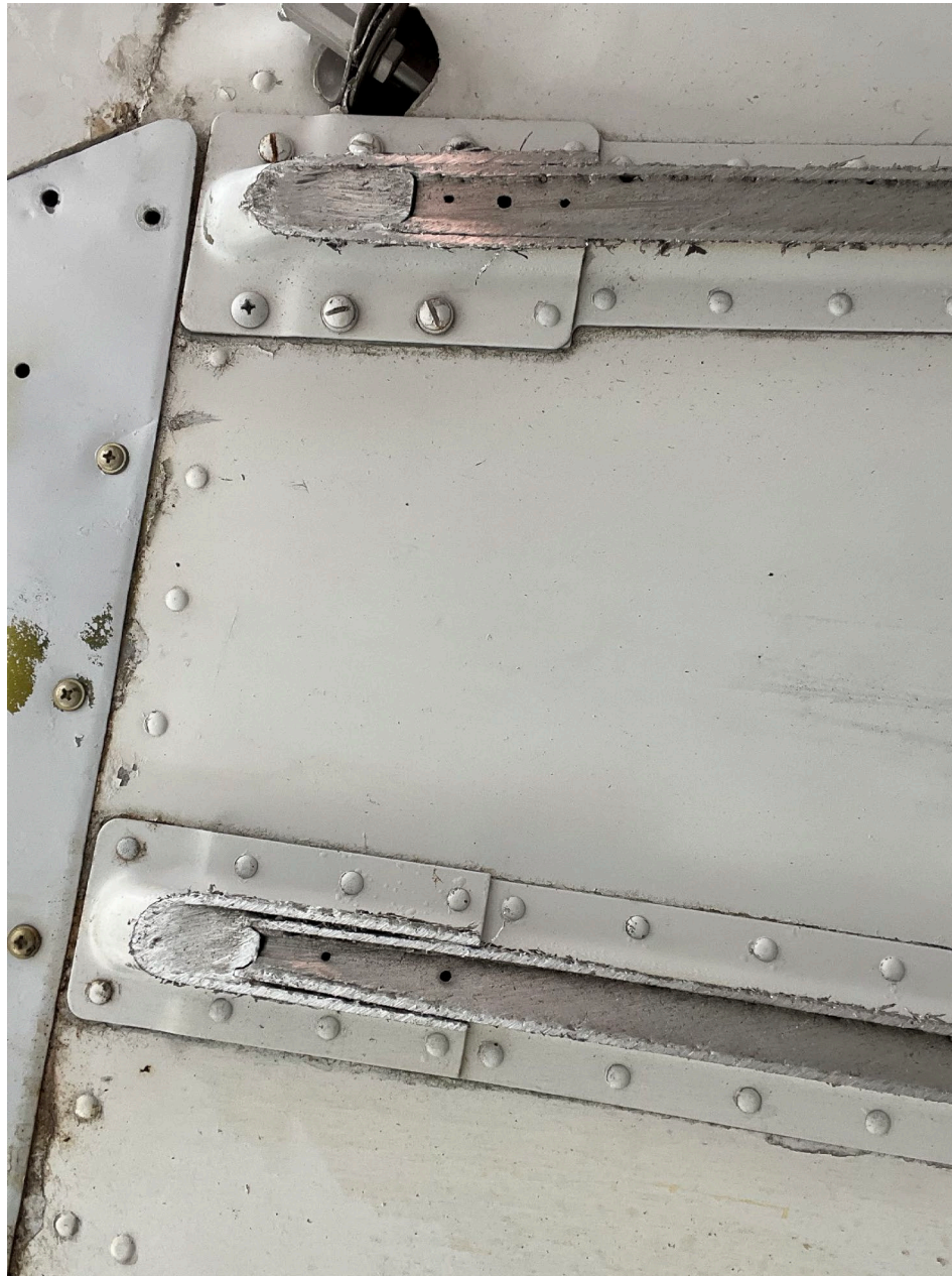
Photo 2 – View of Damage to External Longerons (FAA)
