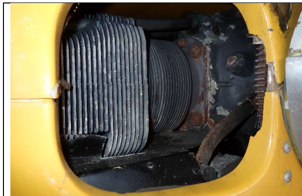
Figure 11: No. 1 Cylinder with visible corrosion at the cylinder base
