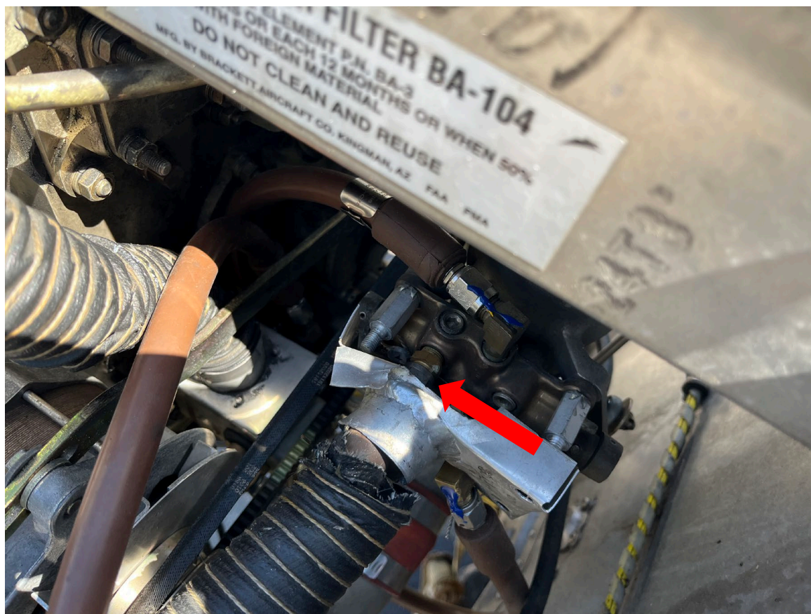
Photograph 3 - Fitting Where the Fuel was Leaking
