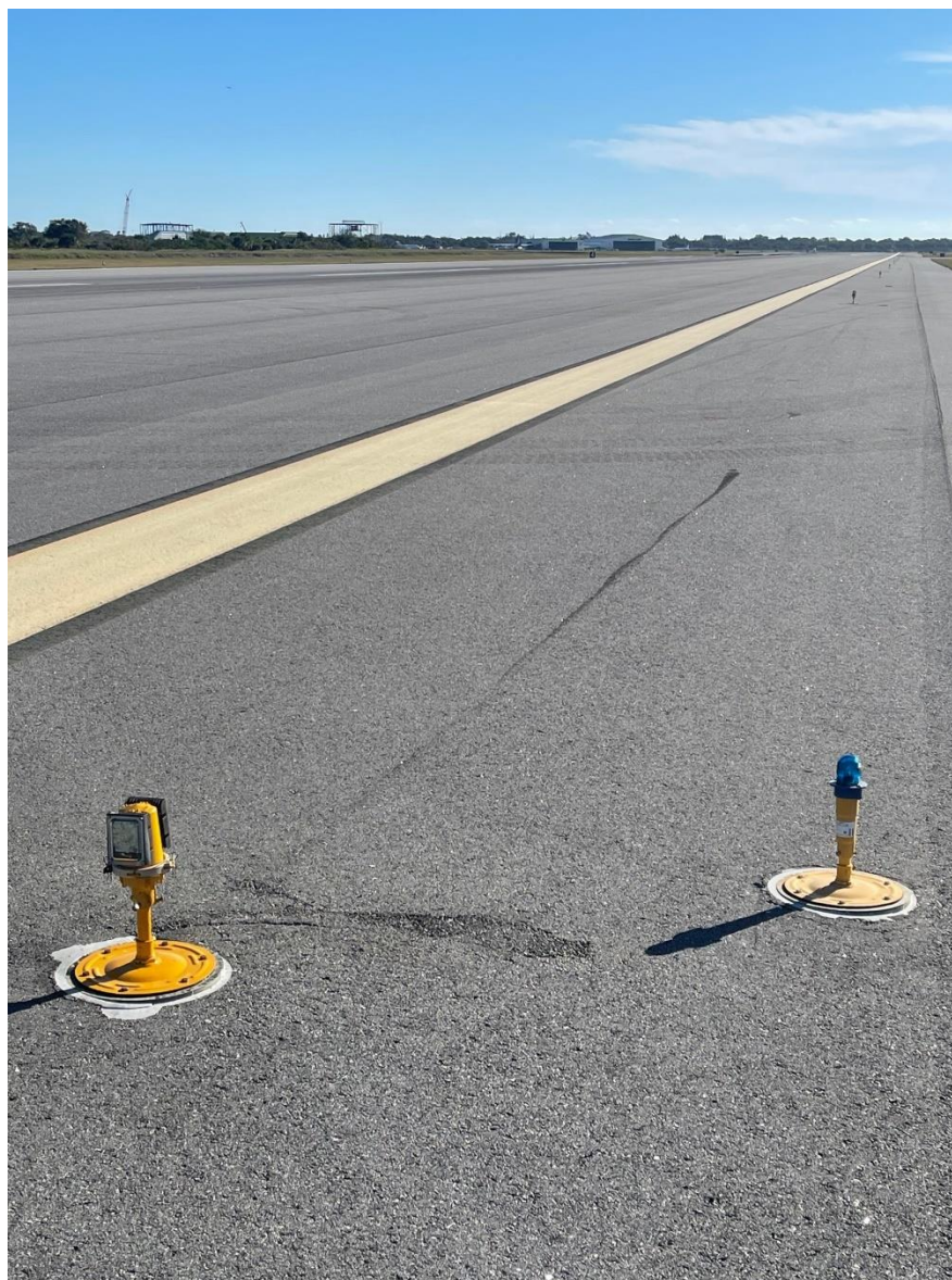
Photograph 2 - Impacted runway light location (Courtesy of FAA)
