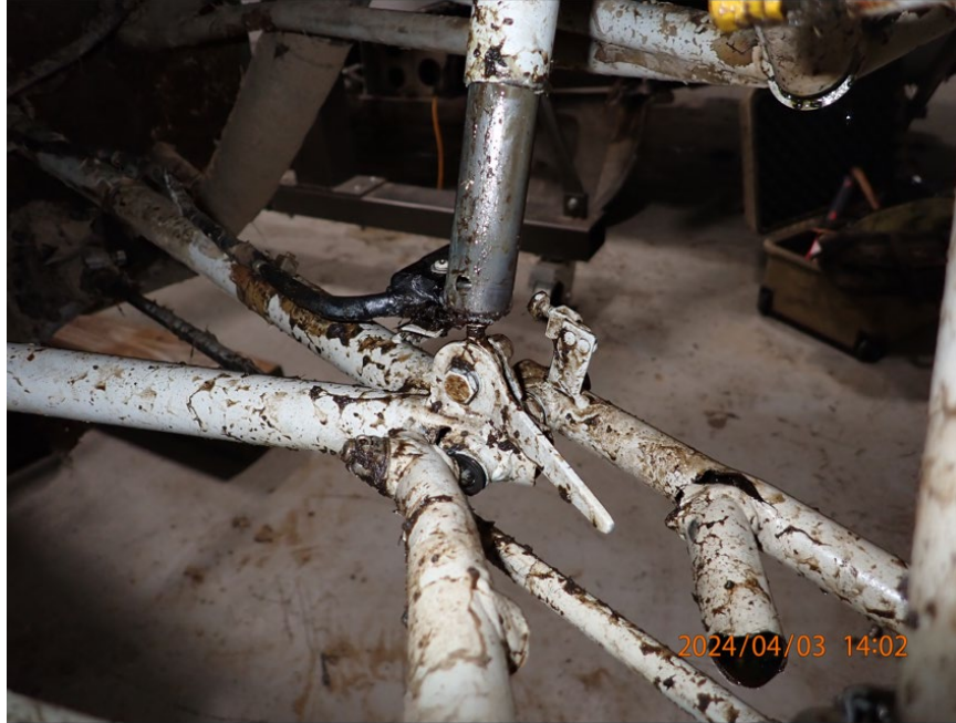
Lower Drag Strut Damage
