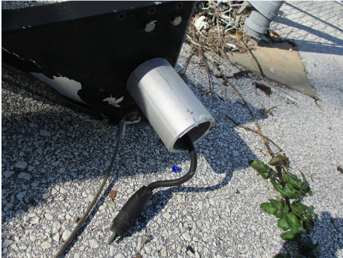
Photograph 10 - View of One Post of the Runway Distance Remaining Sign that Fractured at the Reduced Diameter (Courtesy of FAA)
