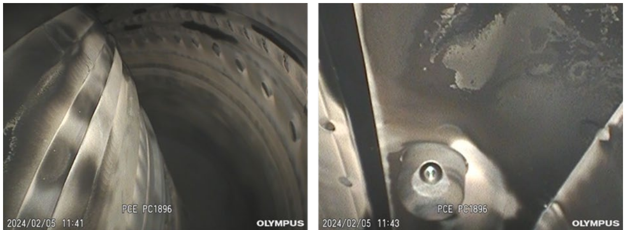
Photo 16- (L) Combustion Liner, (R) Fuel Nozzle
