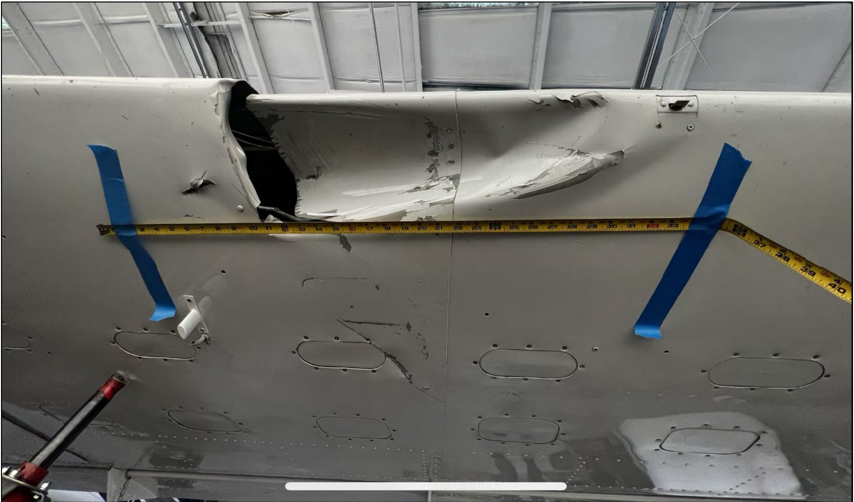
Photo 4: View of the damaged left wing (Photo Courtesy of FAA)
