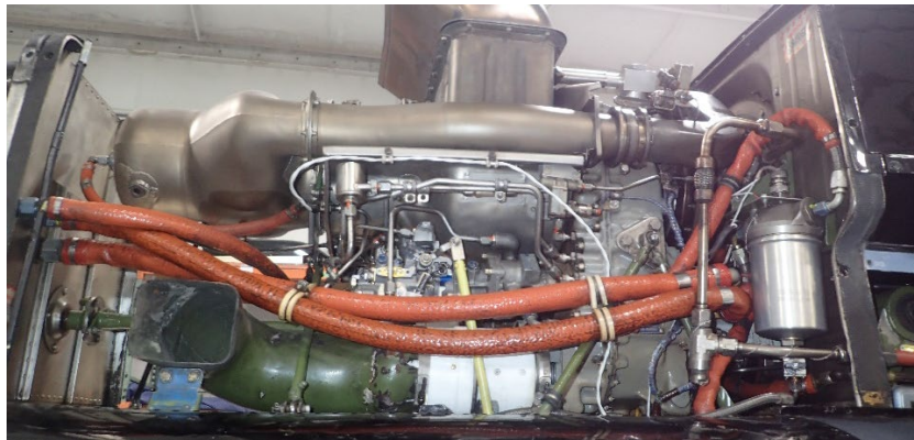
Photo 3 - View of engine and oil supply lines from engine to airframe oil tank.
