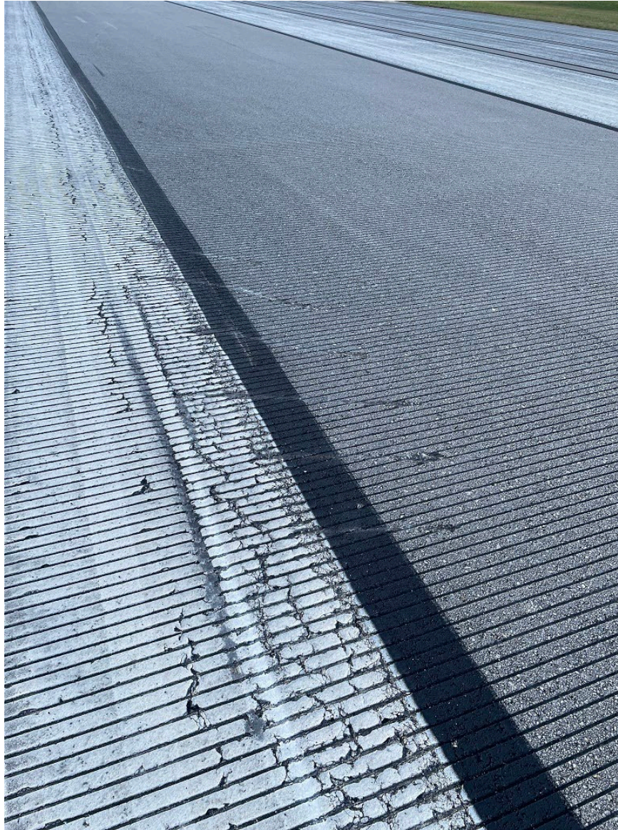
Photograph 4 - Propeller Gouge Marks in Runway (Courtesy of FAA)
