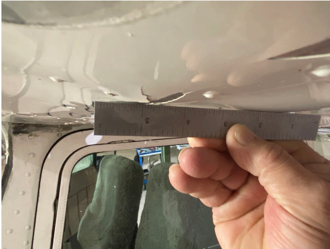
Photograph 2 - Buckling of Left Wing (Courtesy of FAA)
