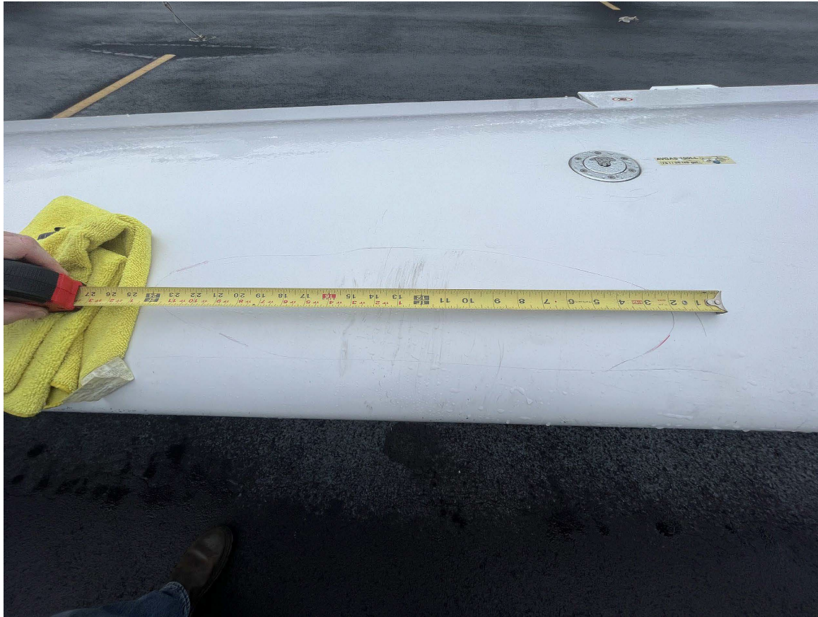
Photograph 1 - Initial damage overview (Courtesy of FAA)
