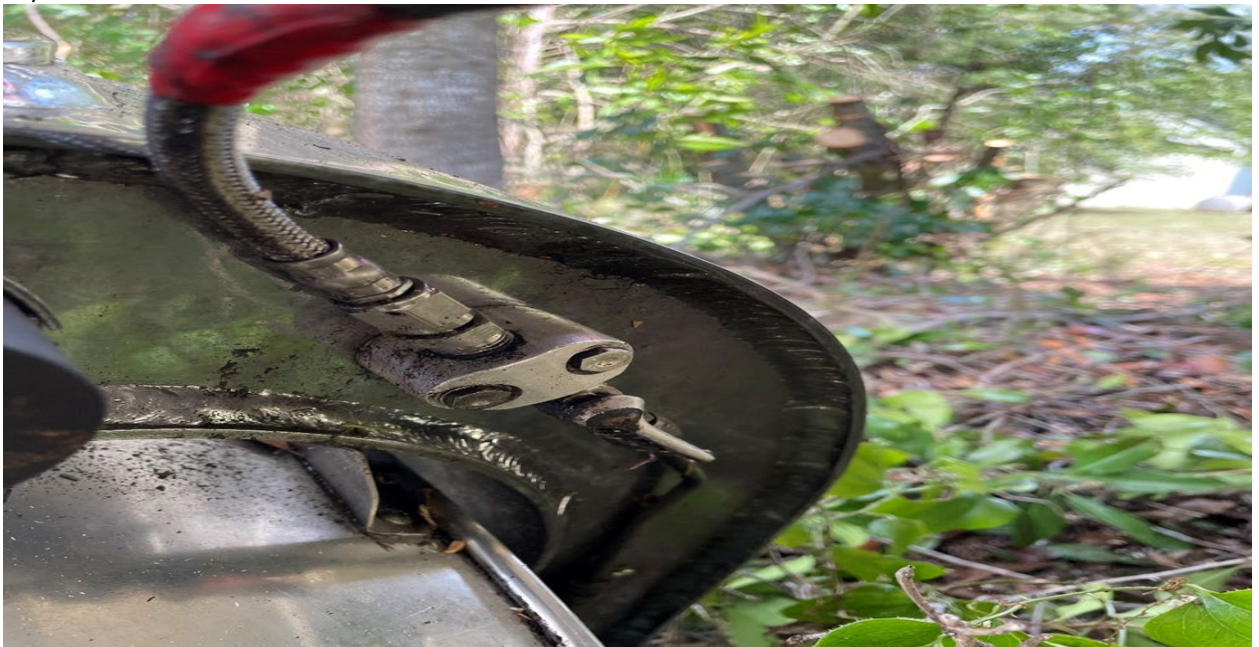
Figure 6. Hydraulic fluid residue
