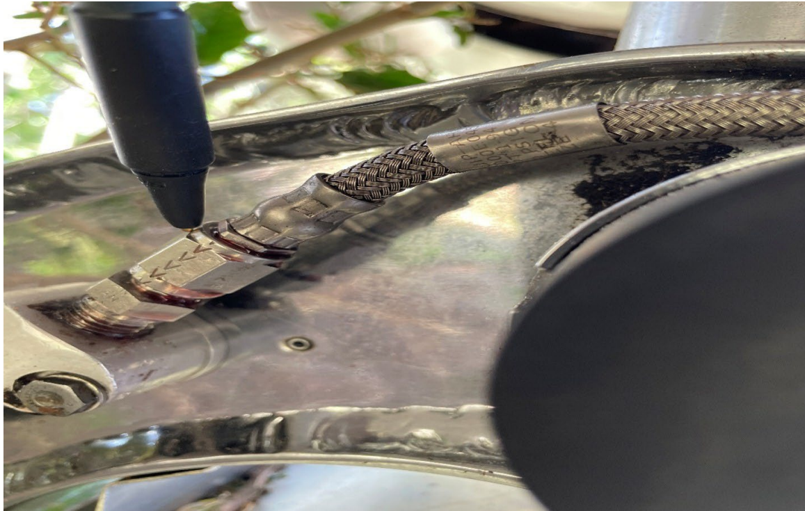
Photograph 4 - Close up view of loose B-Nut fitting hydraulic fluid leakage.
