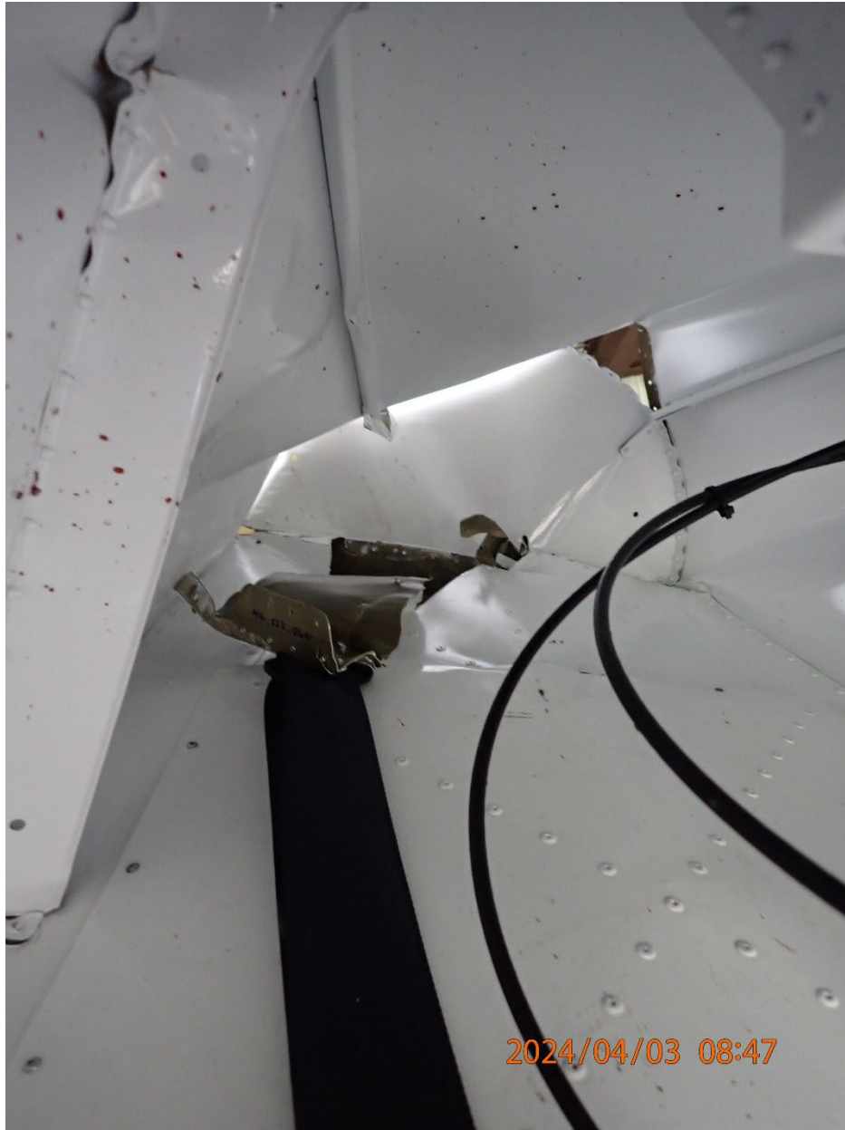
Photo 19: View of the shoulder harness attachment point pulled from the airframe.
