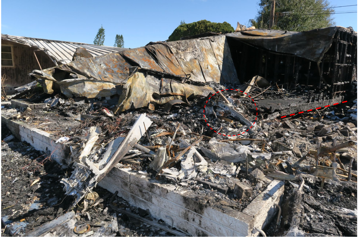
Figure 2. Aircraft wreckage location. Red dashed circle denotes the location of the engine. Red dashed line runs parallel to the rim joist of the manufactured home showing its displacement with respect to the brick foundation.
