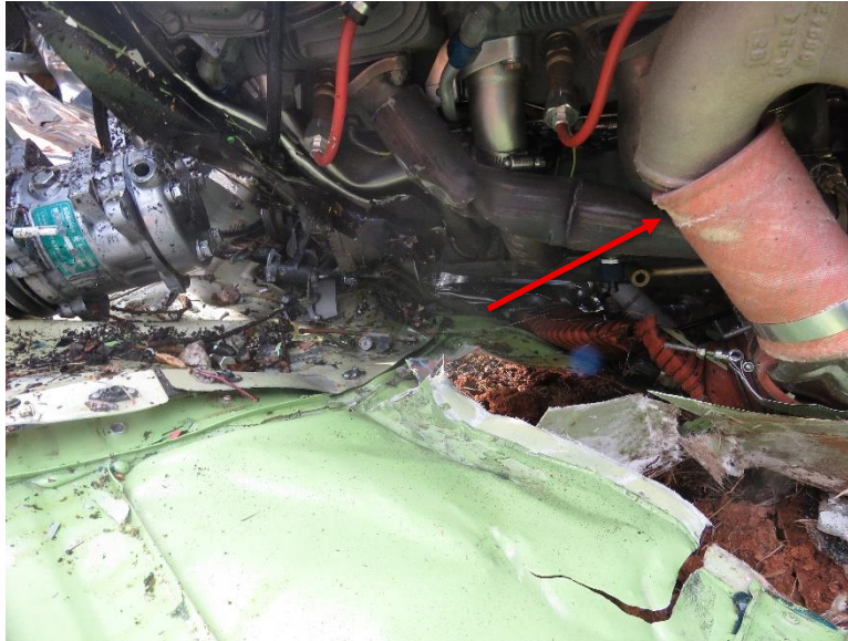
Photo 36 - Left side intercooler hose with missing clamp, with arrow pointing to clamp location (Photo Source: Lycoming Engines)
