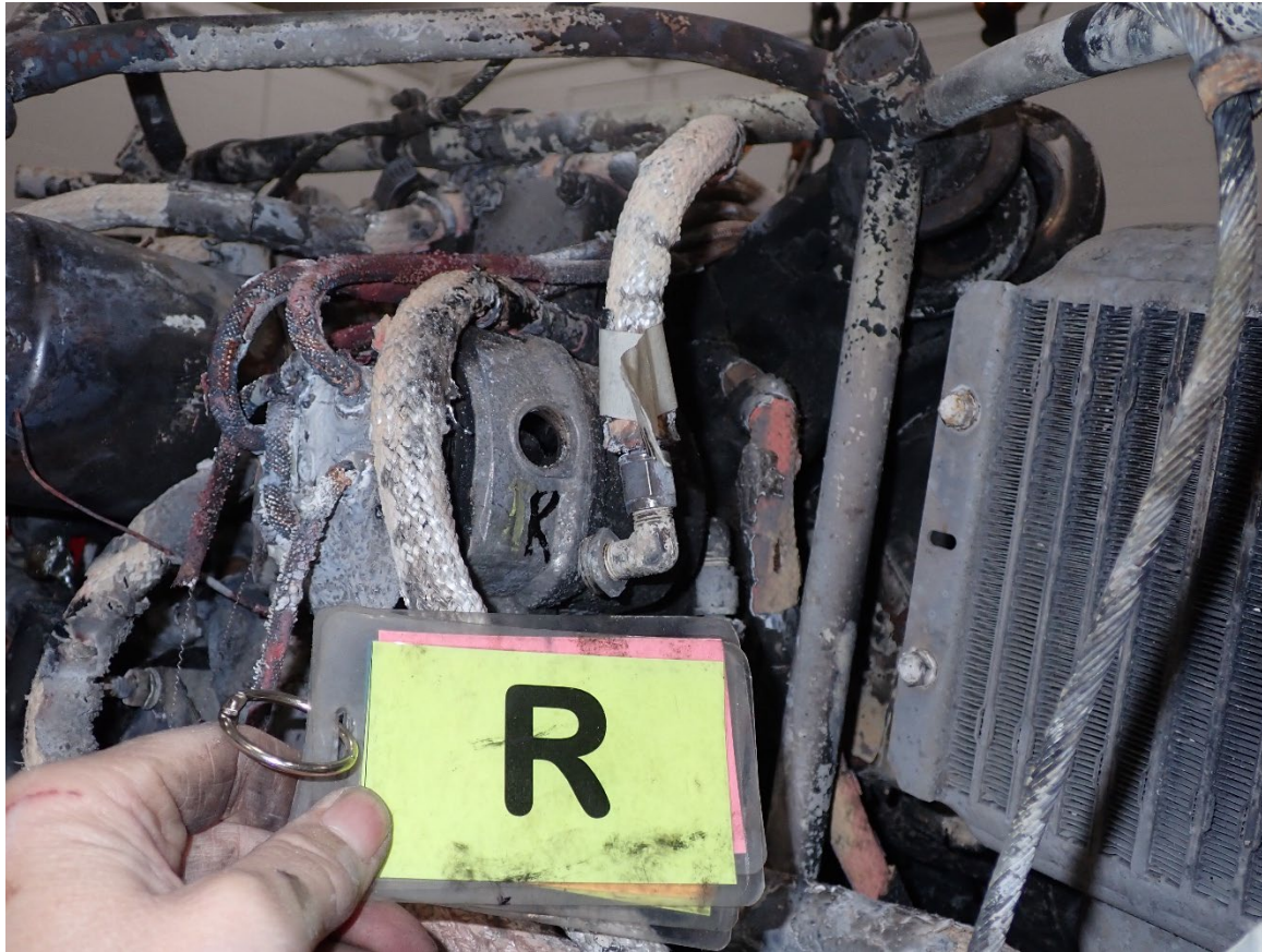
Photograph 14 - NTSB Digital Photograph. View of Heat Damaged Right Magneto
