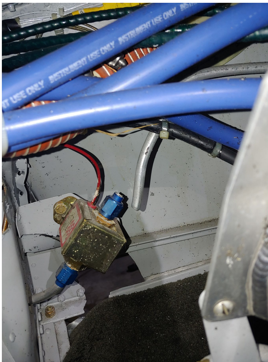
Photograph 7 - View of boost pump with fractured fuel line. (Courtesy of FAA)
