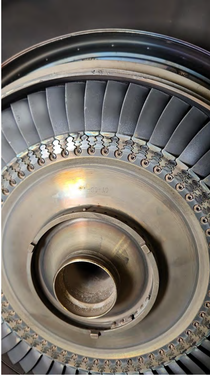
CT blades were turned with starter gen outlet and free to spin no rubbing or noises. Back of CT blades show evidence of rubbing on inter baffle section vane
