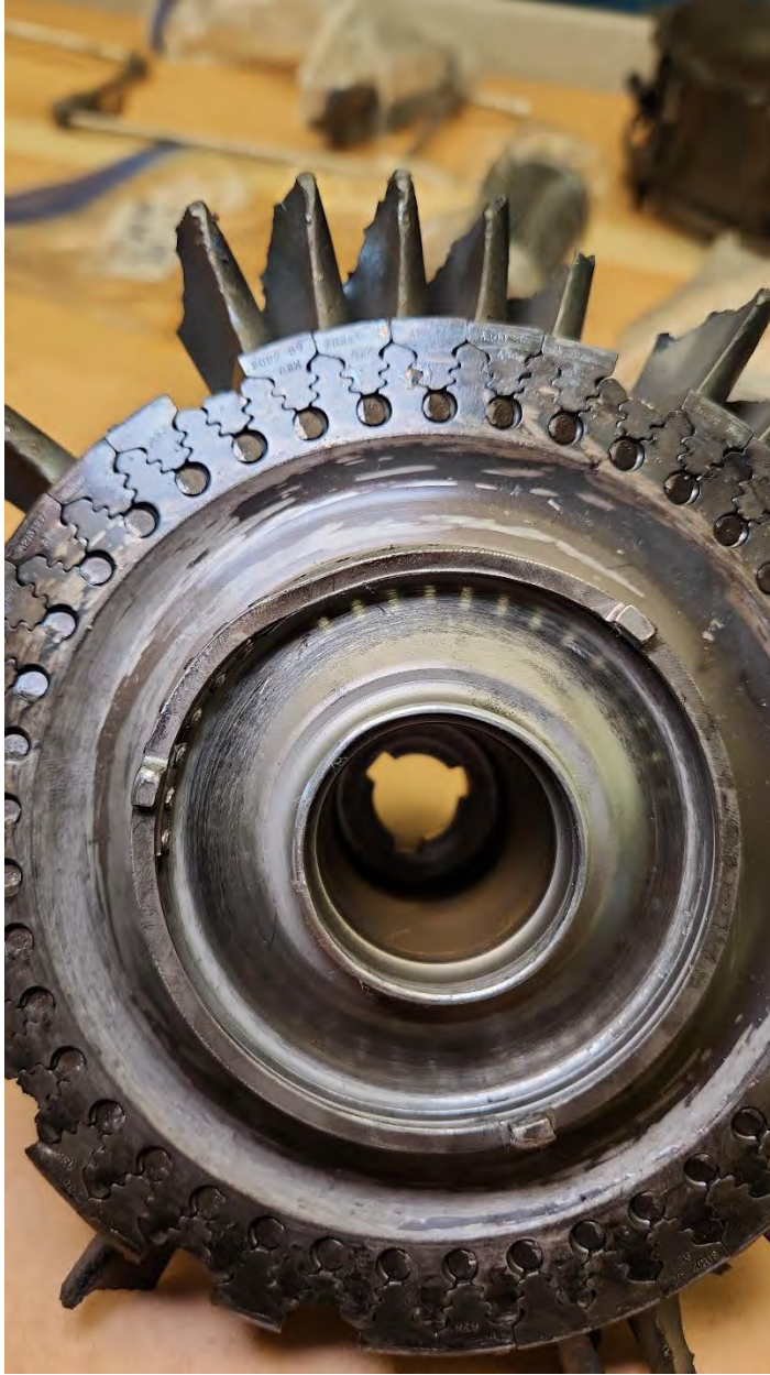
PT Wheel deformation
