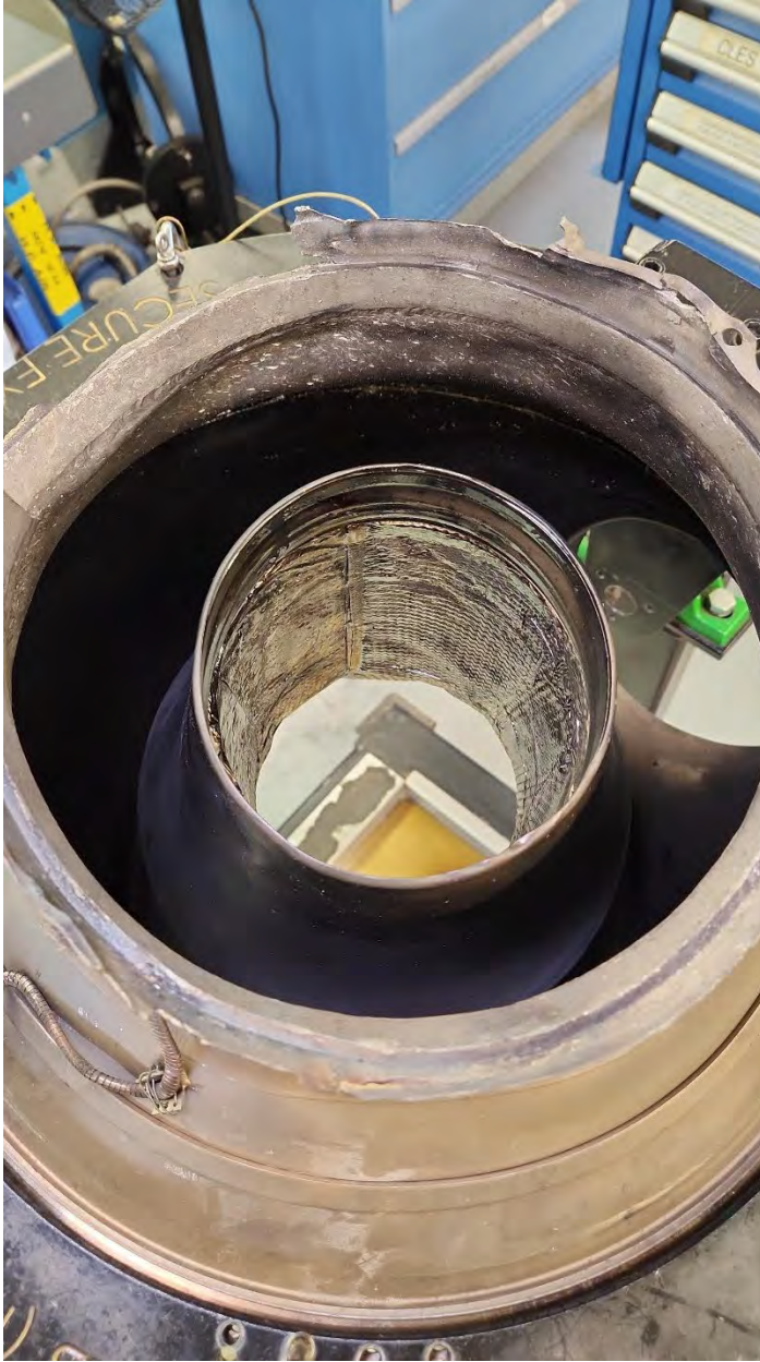
Exhaust Casing liner found offset
