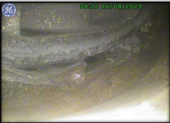
23. Power Turbine Stator and Housing. Damaged from Blade failure.
