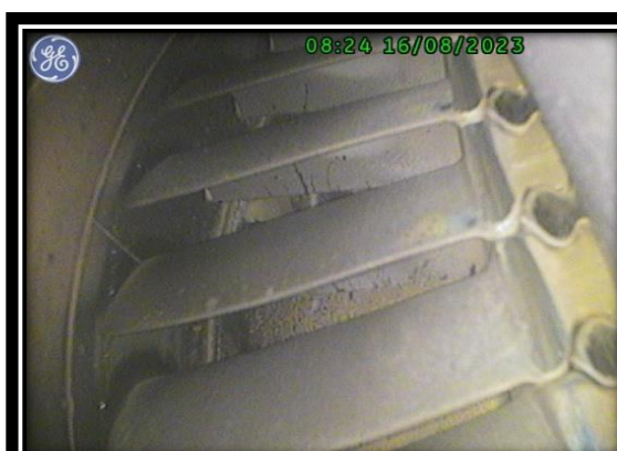
16. Compressor Turbine Blades. Showing signs of light rub and soot from a fire in the gas path post shutdown.
