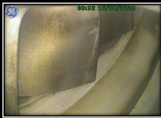
8. Signs of light to moderate rub on First Stage Compressor. Bottom/Gravity side.
