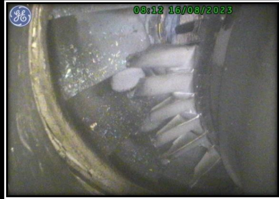
22. Power Turbine Blades. Heavily damaged, with breakage.
