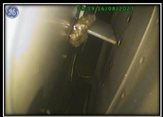
20. Picture of debris in the gas case, at diffuser tubes.
