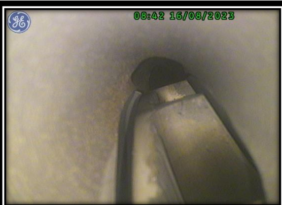
10. Centrifugal Compressor Disc. No signs of damage.
