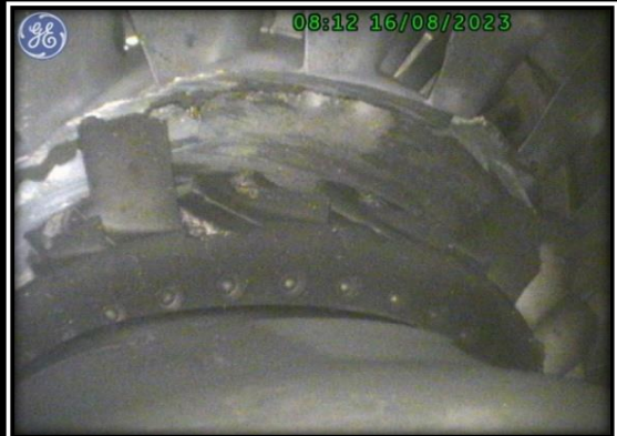
24. Power Turbine Blades and Disc. Complete Blade failure at the root/fir tree.
