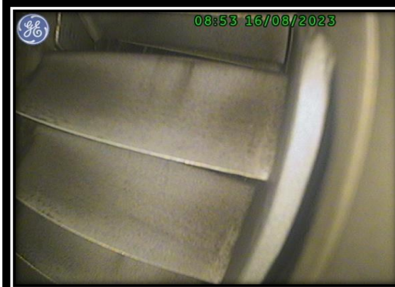
12. Centrifugal Compressor Guide Vanes
