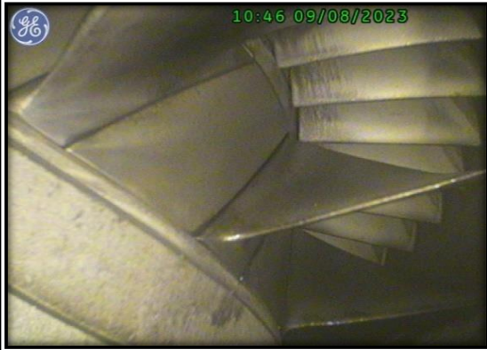
5. First Stage Compressor. Showing signs of very fine erosion.
