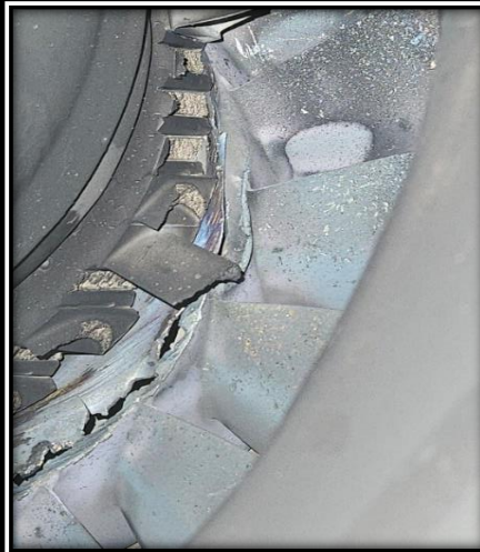
26. PT Blade breakage at root/fir tree.
