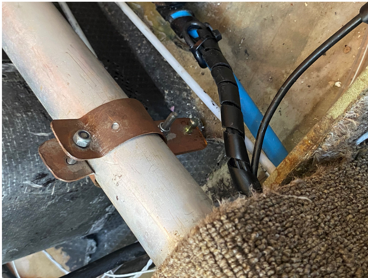
Photo 4: View of the autopilot servo bracket on the elevator control tube. (Photo Courtesy of FAA)
