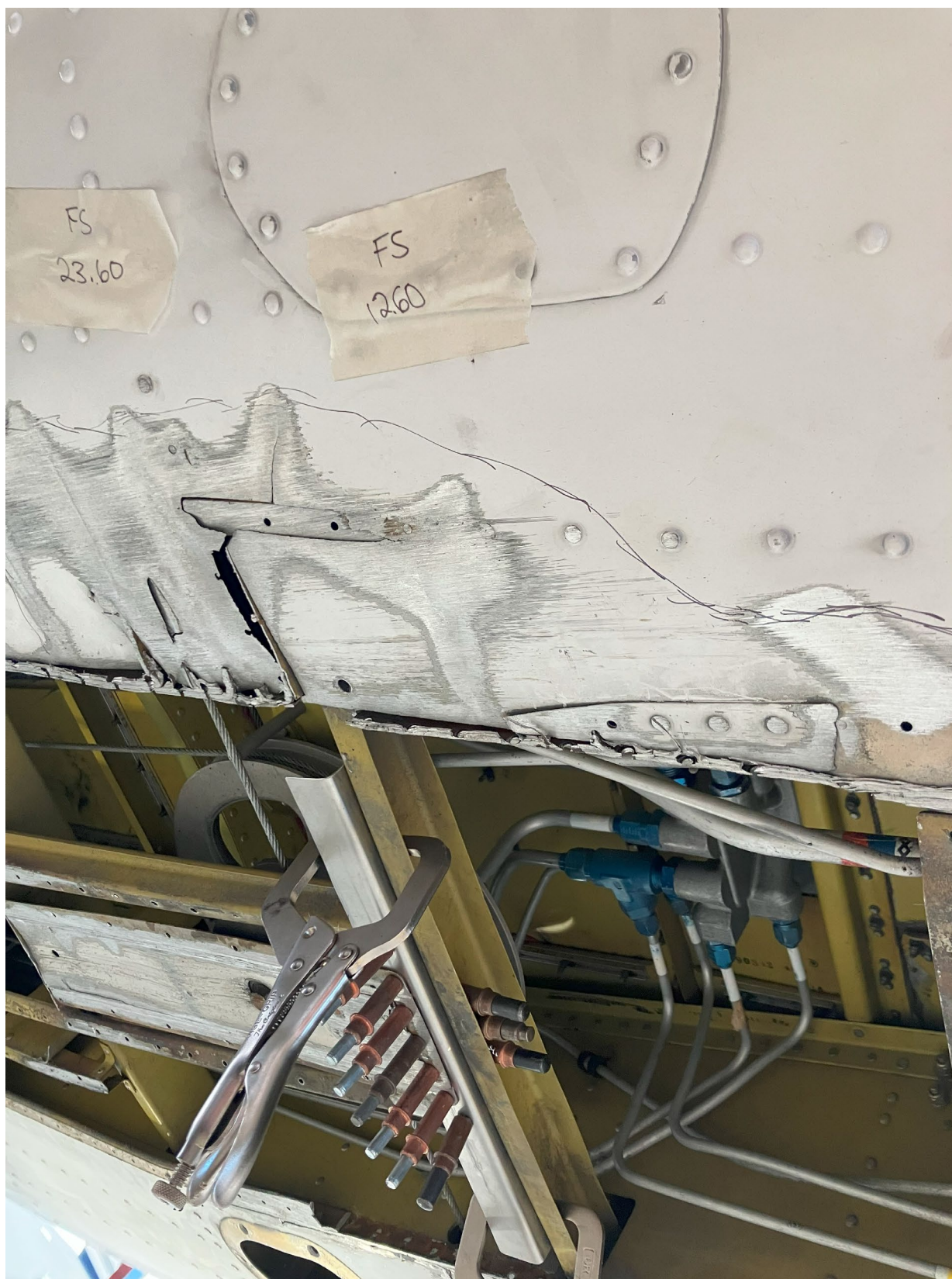
Figure 5 Repair angle at FS23.5, and chafed skin RH Side
