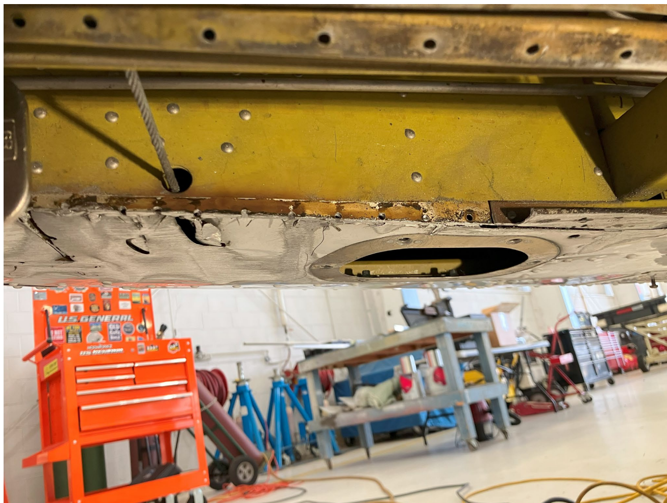
Figure 3 Chafed skin been trimmed out LH Side aft of FS23.5
