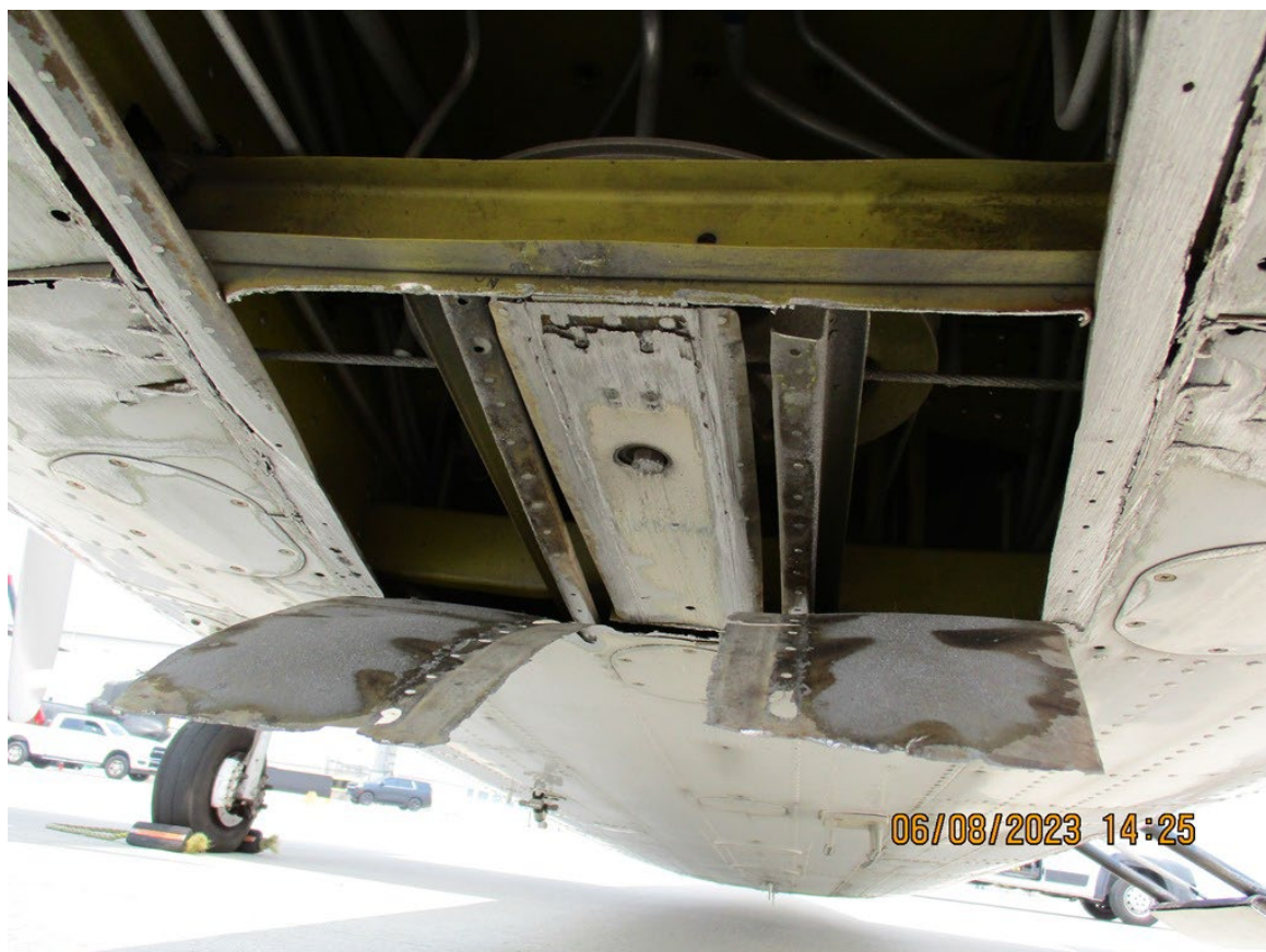
Photograph 1 - Damage aft of nose gear landing well (Courtesy FAA)
