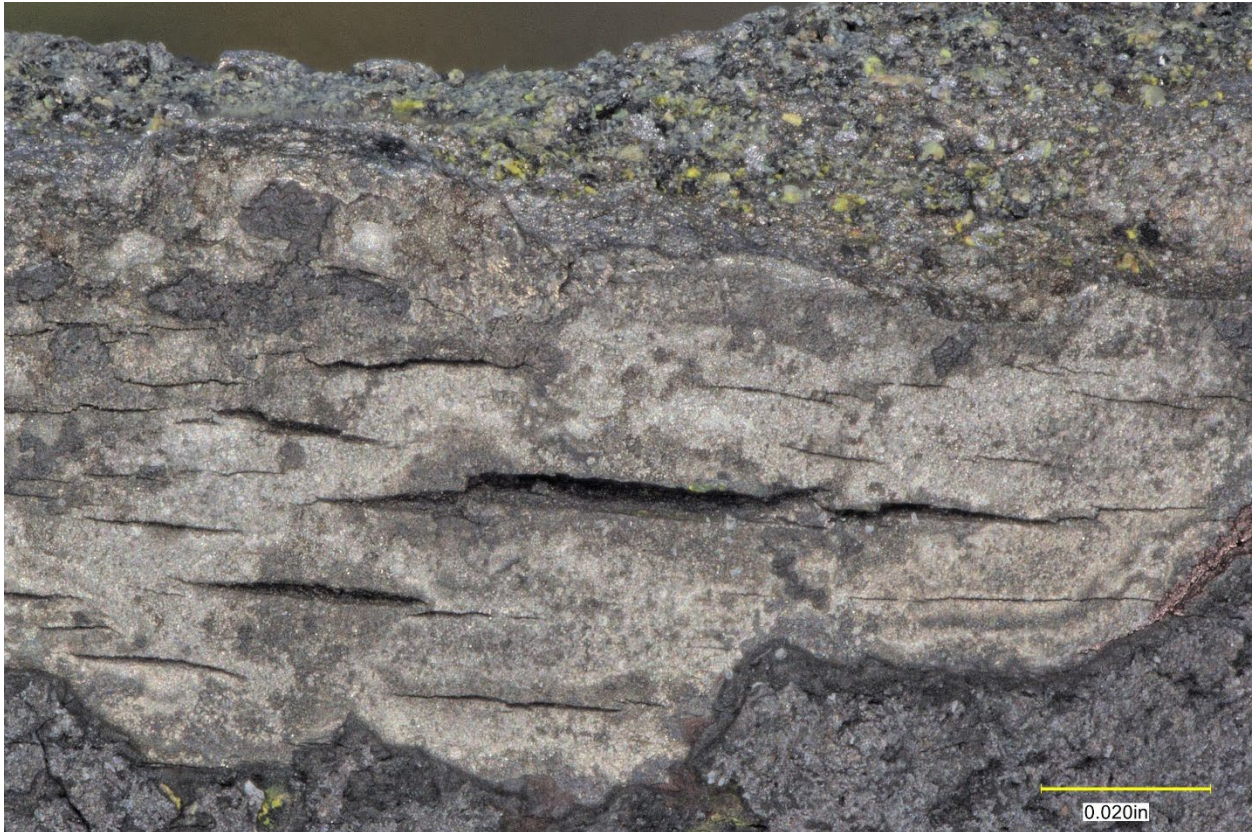
Figure 15. Closer view of the parallel cracks in Figure 14.
