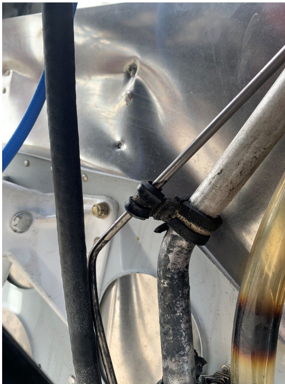
Photo 2 – View of firewall damage (photo courtesy of FAA)
