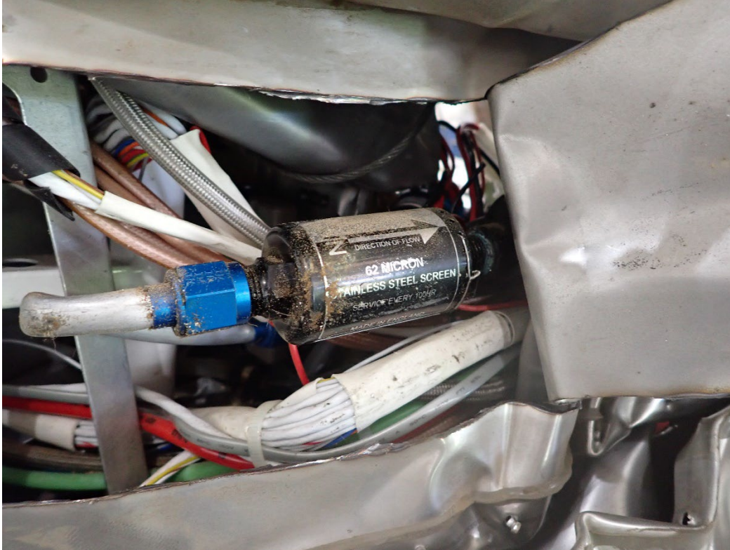
Photo 35: View of the inline fuel filter.
