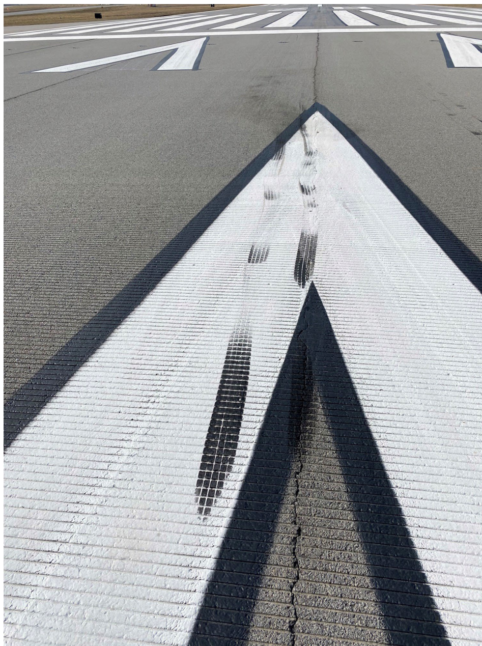
Photo 1 – View of Ground Scars and Rubber Transfer Marks Consistent with Left Main Landing Gear (FAA)
