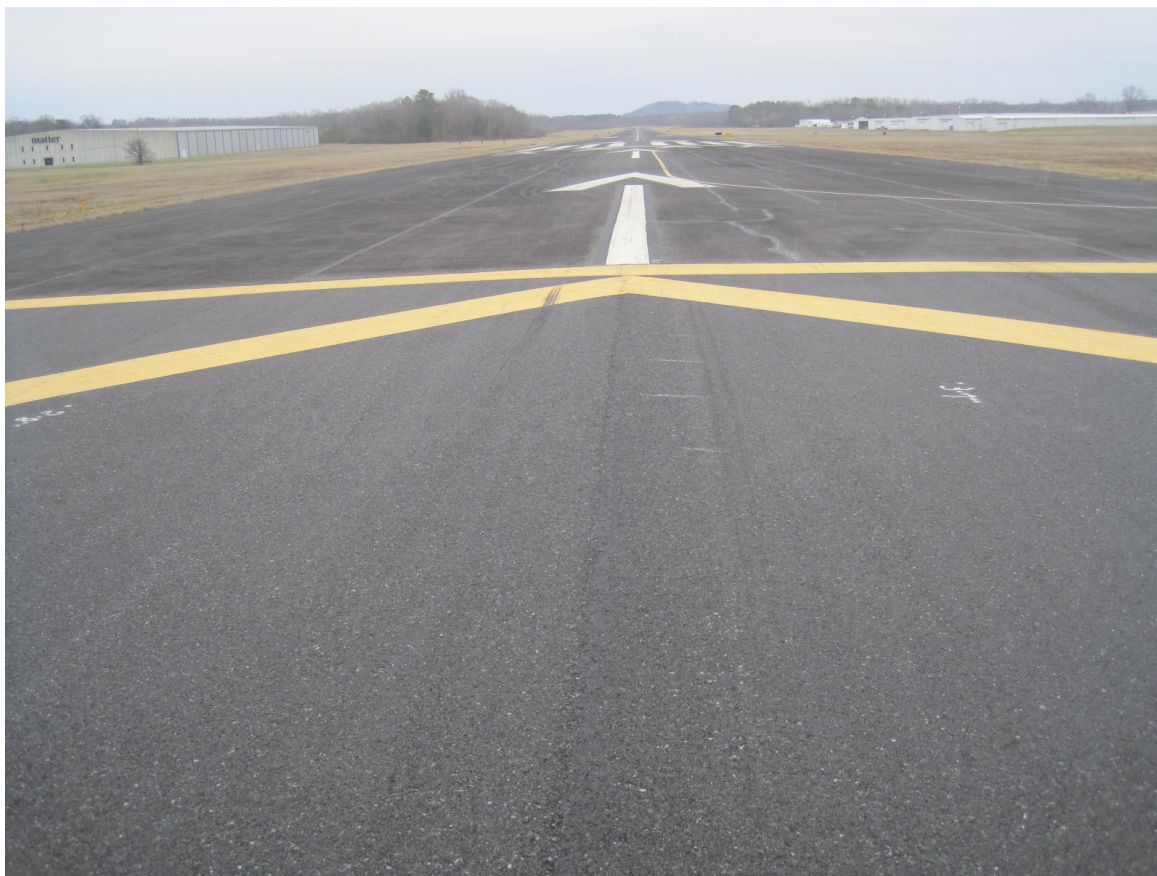
Photograph 1 - Propeller Strike Marks on Displaced Threshold (Courtesy of FAA)
