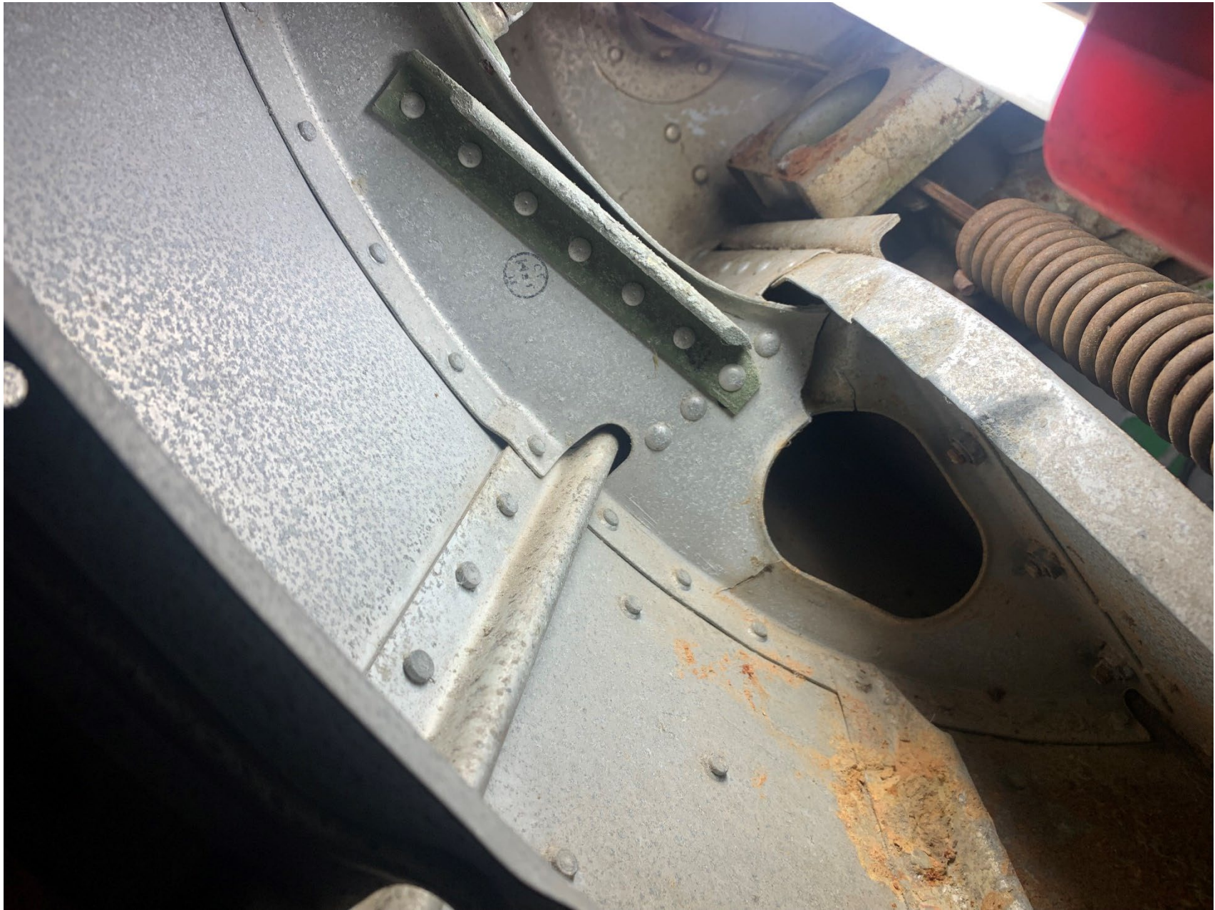
Photo 3 – cracked stringers (FAA)
