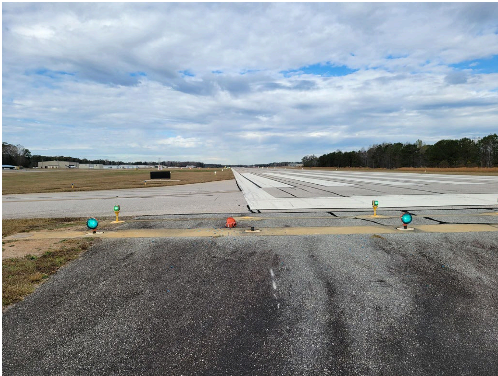
Photo 1 – Damaged Runway Light (Photo Courtesy of FAA)
