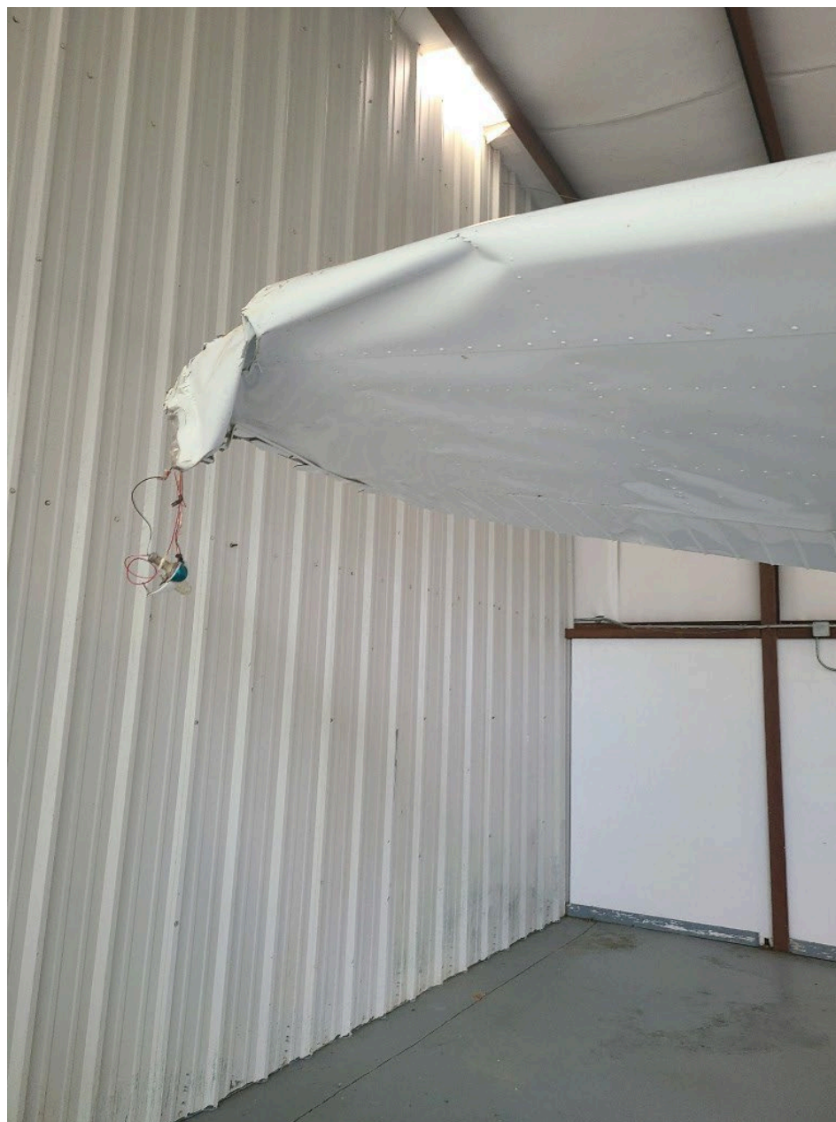
Photo 2 - Damage to Right Wing Spar (FAA)
