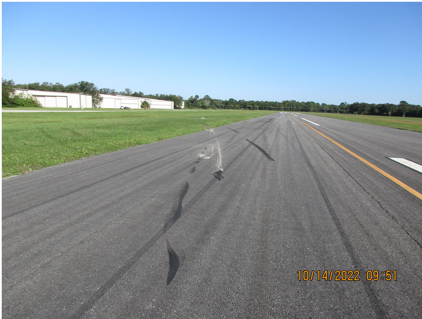
Photo 1 – FAA Digital Photograph. View Showing the Impact on the Runway.
