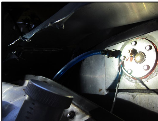
Figure 4: View of the Fuel Sender Unit.
