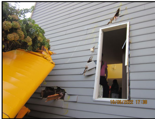
Figure 5: View Showing Damage to House.
