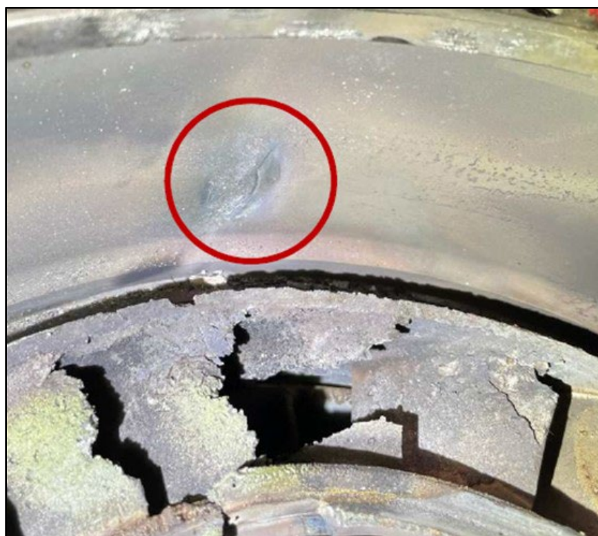
Figure 30. PT Containment Shield - Impact Mark
