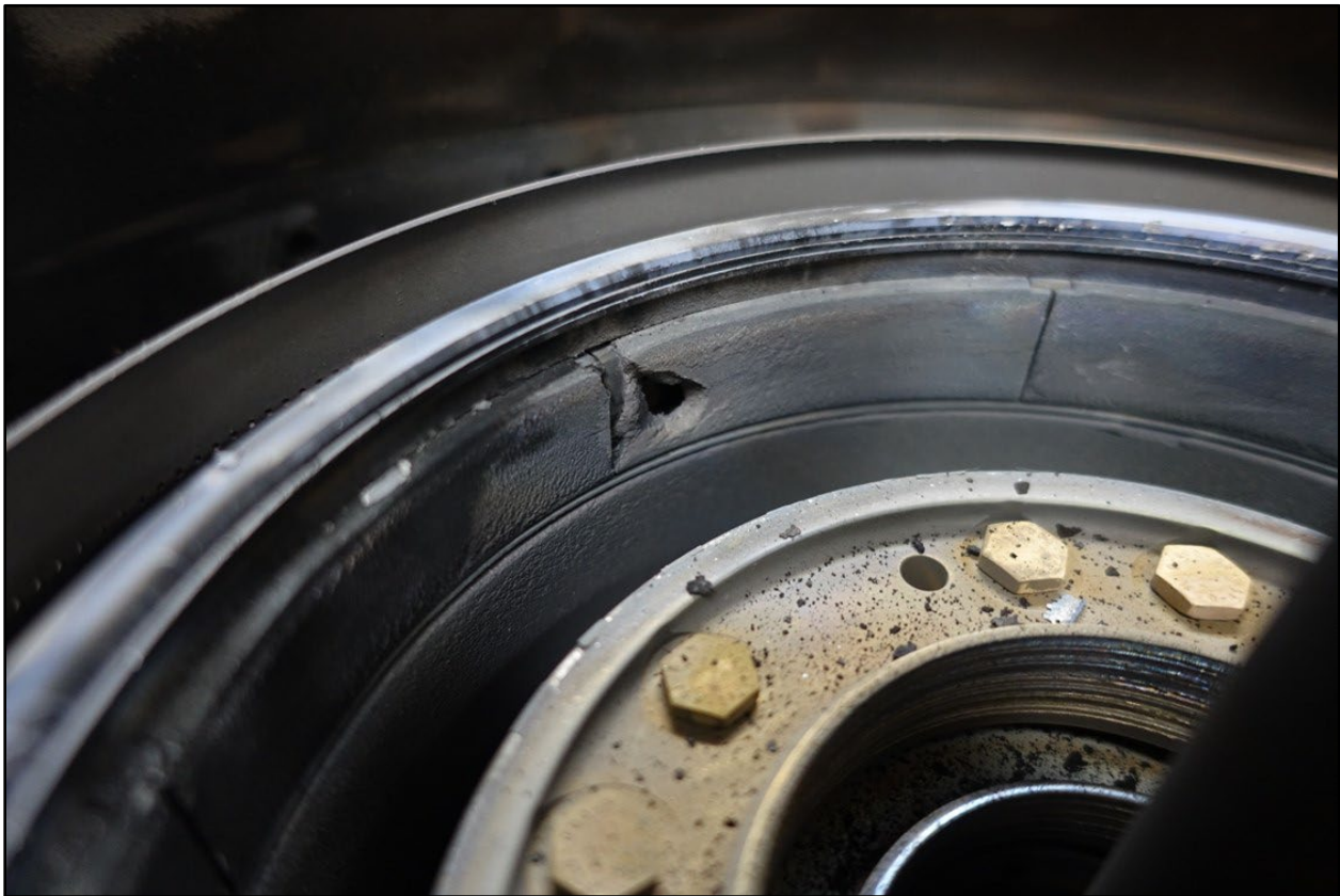
Figure 24. Gas Generator Turbine Shroud - Missing Material
