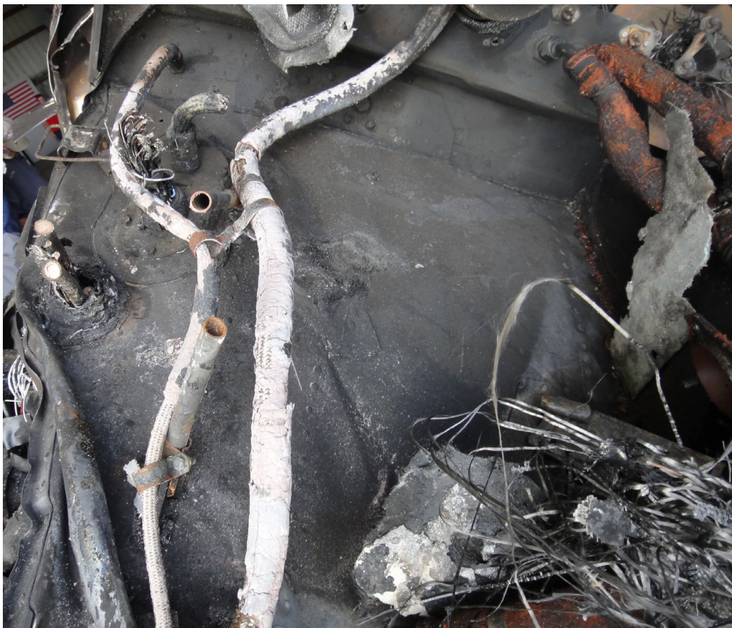
Figure 8. Photograph of engine #1 inboard firewall.
