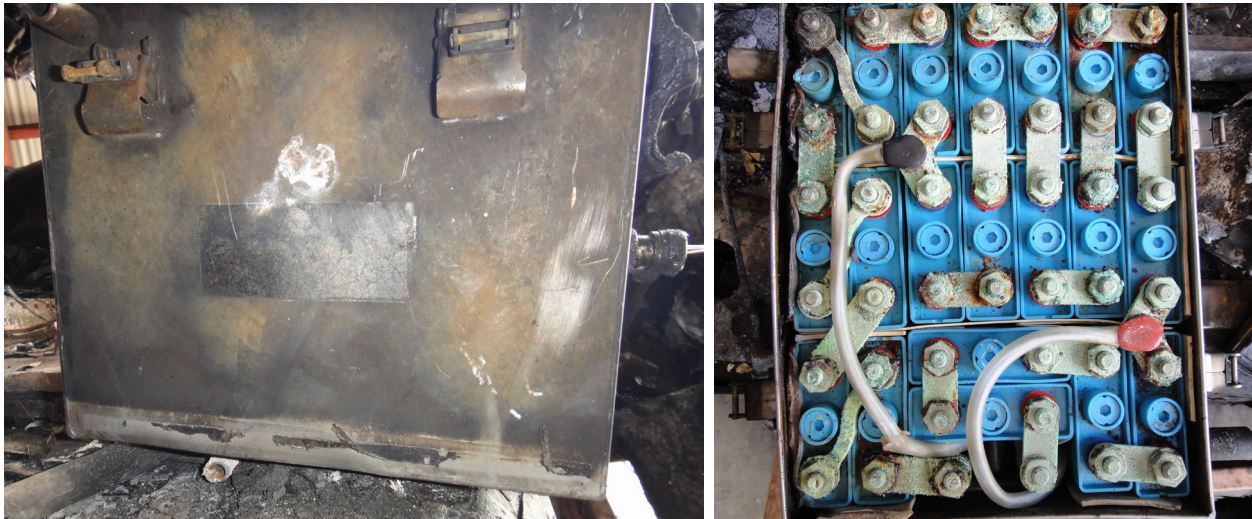
Figure 7. Photograph of aircraft battery case (left) and interior (right).
