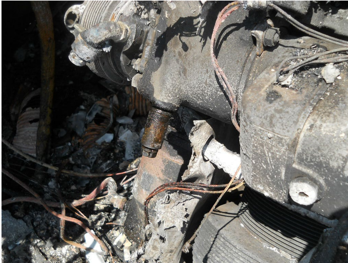
Photograph 6 - Loose Oil Sump Accessory Port Plug
