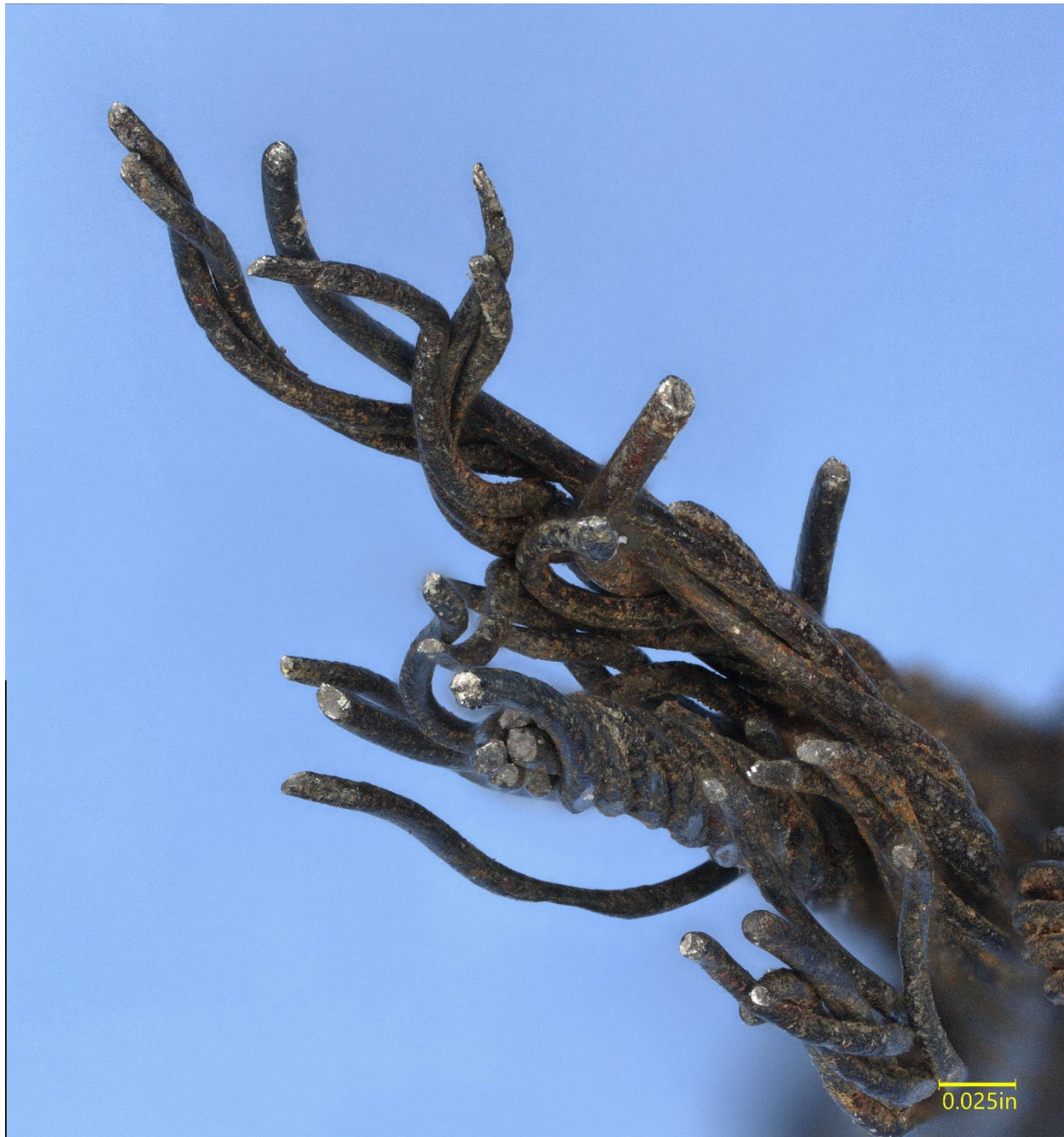
Figure 6 End 2 Fracture Surfaces S (40X). View Showing the Ends of the Fractures Strands
