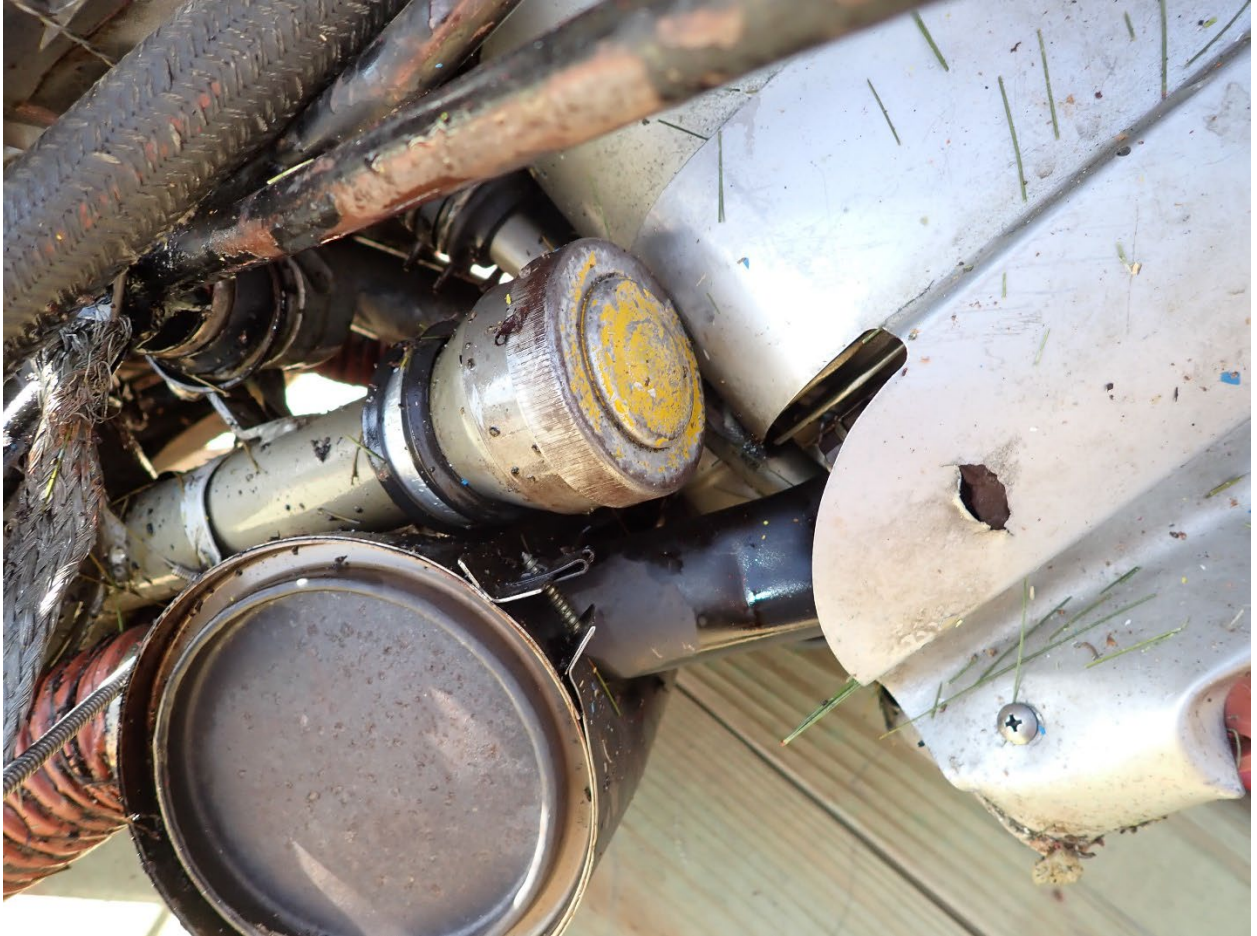
Figure 30: Oil fill cap secured to the engine
