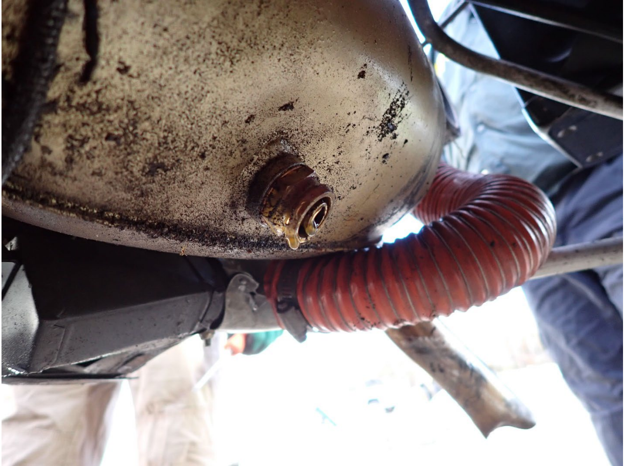
Figure 9: Broken oil quick drain
