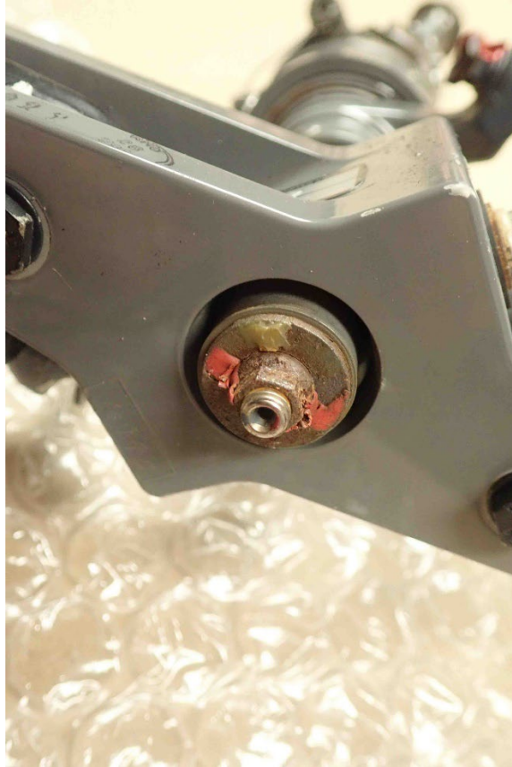
Figure 1 – Corrosion to hardware
