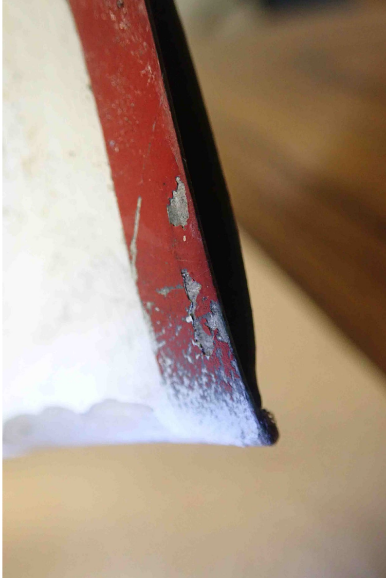
Figure 9 – Corrosion and paint bubbles
