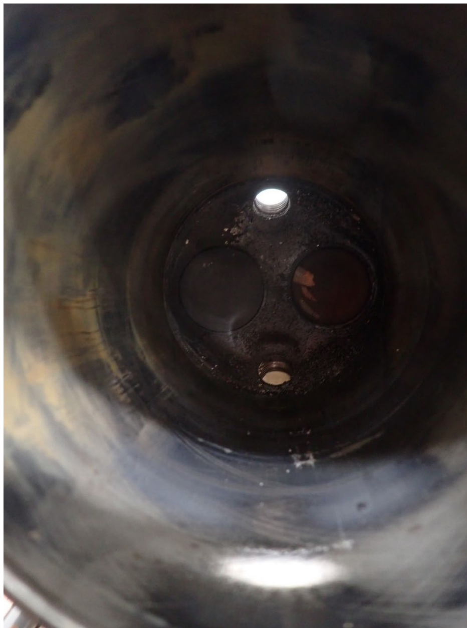
Photo 3 – View of the interior of cylinder No. 4, the exhaust valve on the right and remained in the closed position.
