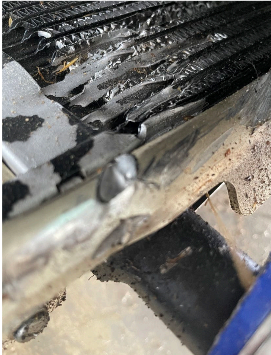
Photo 5 – Damaged radiator. Impact damage from drive flange parts. (Courtesy of FAA)
