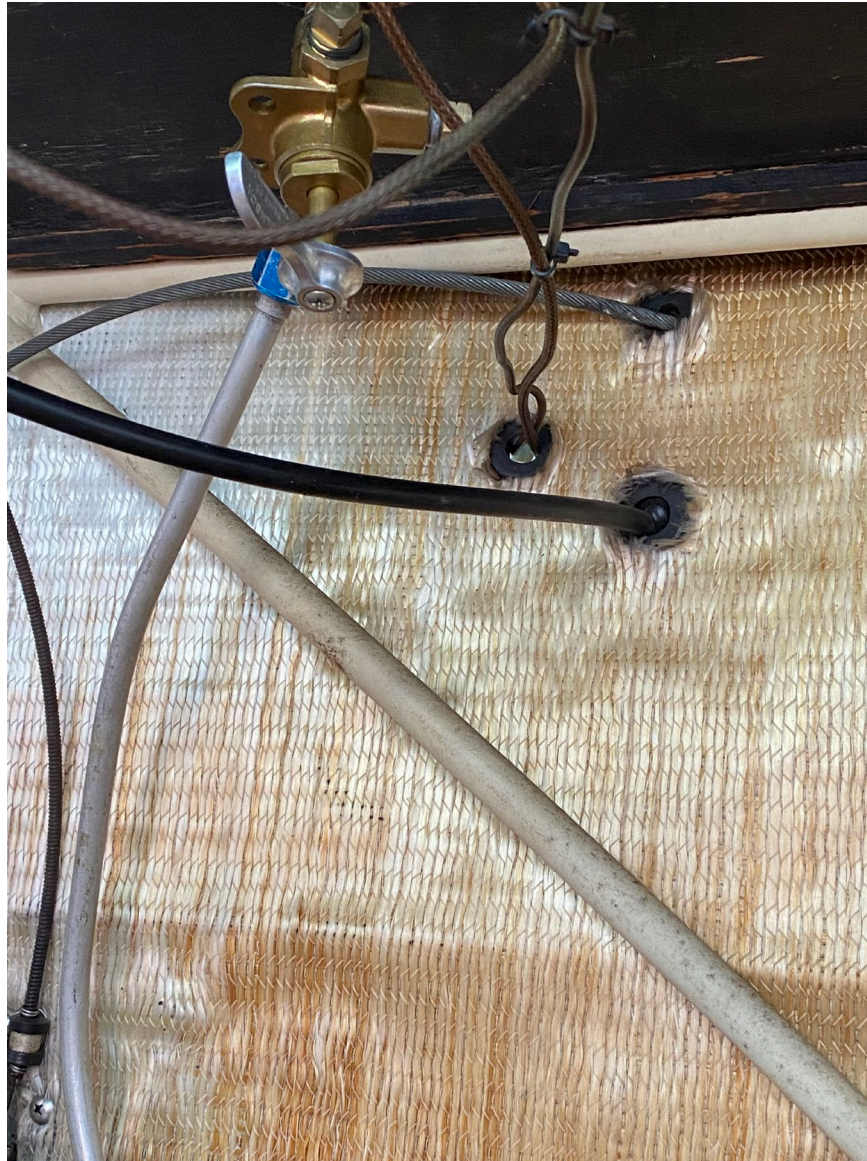
Photograph 6 - Header tank fuel shutoff valve (Courtesy of FAA)
