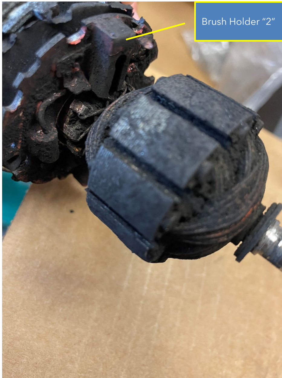
Figure 8 - Main Pump Motor - Brush Holder 2
