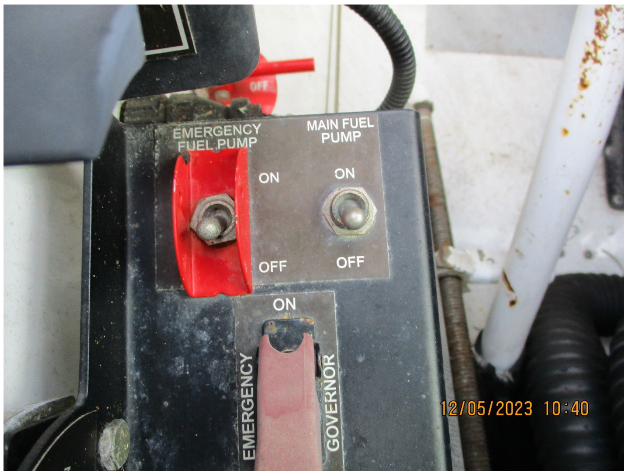
Figure 2 - Fuel Pump Switches
