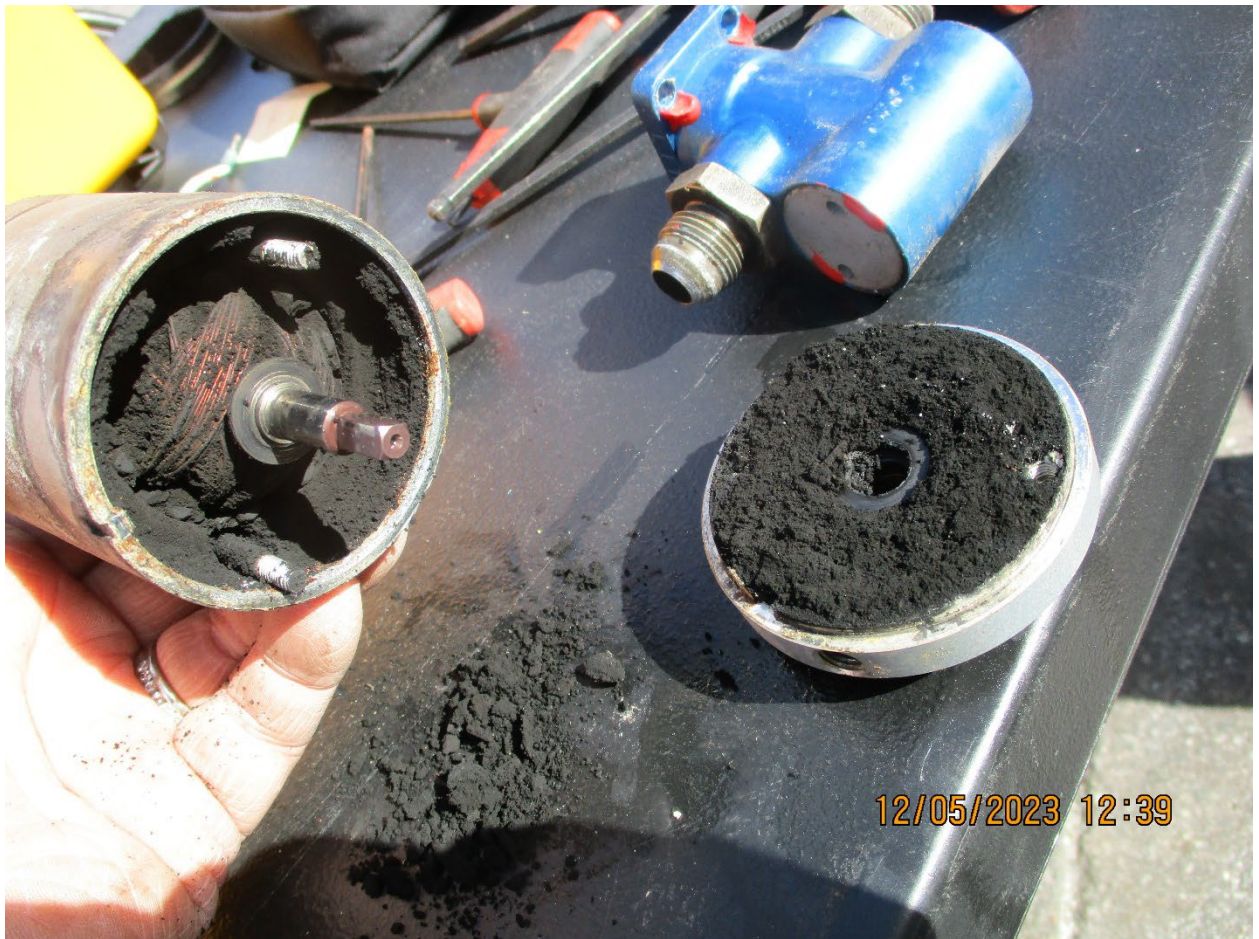
Figure 6 - Main Pump Motor (End Removed)
