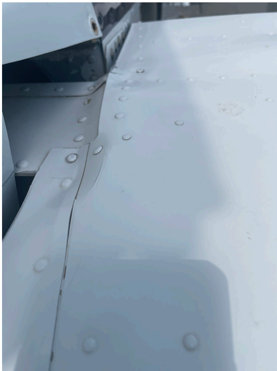
Photo 4 – FAA Digital Photograph. View Showing the Structural Damage to the Right Side of the Stabilator.
