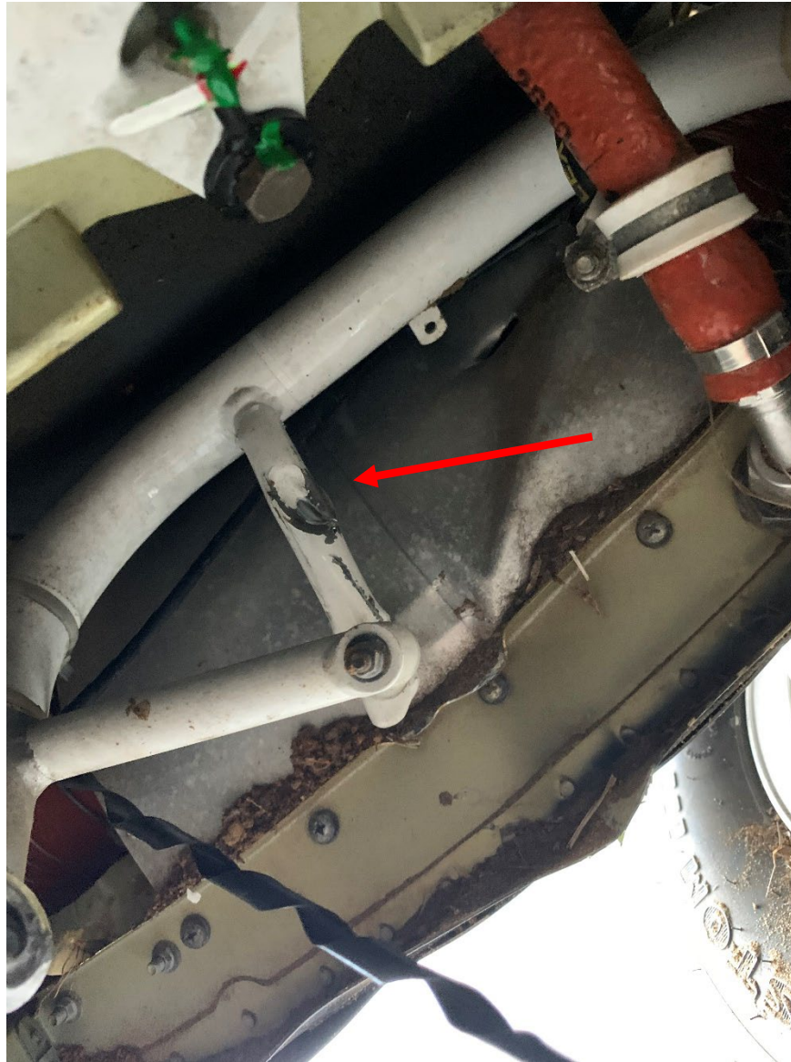
Photograph 4 - Damage to Engine Mount Structure (Courtesy FAA)
