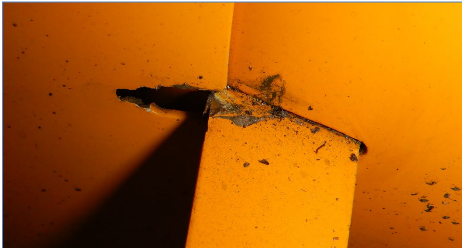
Photo 13 - Close-up view of left rudder horn and empennage damage
