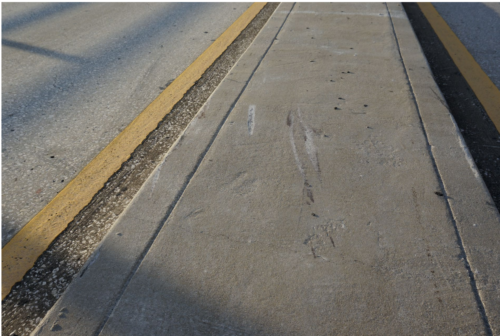
Photograph 5 - Witness Marks on Median
